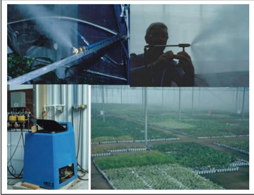
Figure 4. Fog systems form fine water droplets with an average size of 15 \mu\text{m} . Fog has a high surface: volume ratio, which helps water remain suspended in air as a vapor (gas) to maximize evaporation. Fog does not condense, avoids over-saturation of media and foliar leaching, which occurs with mist.
