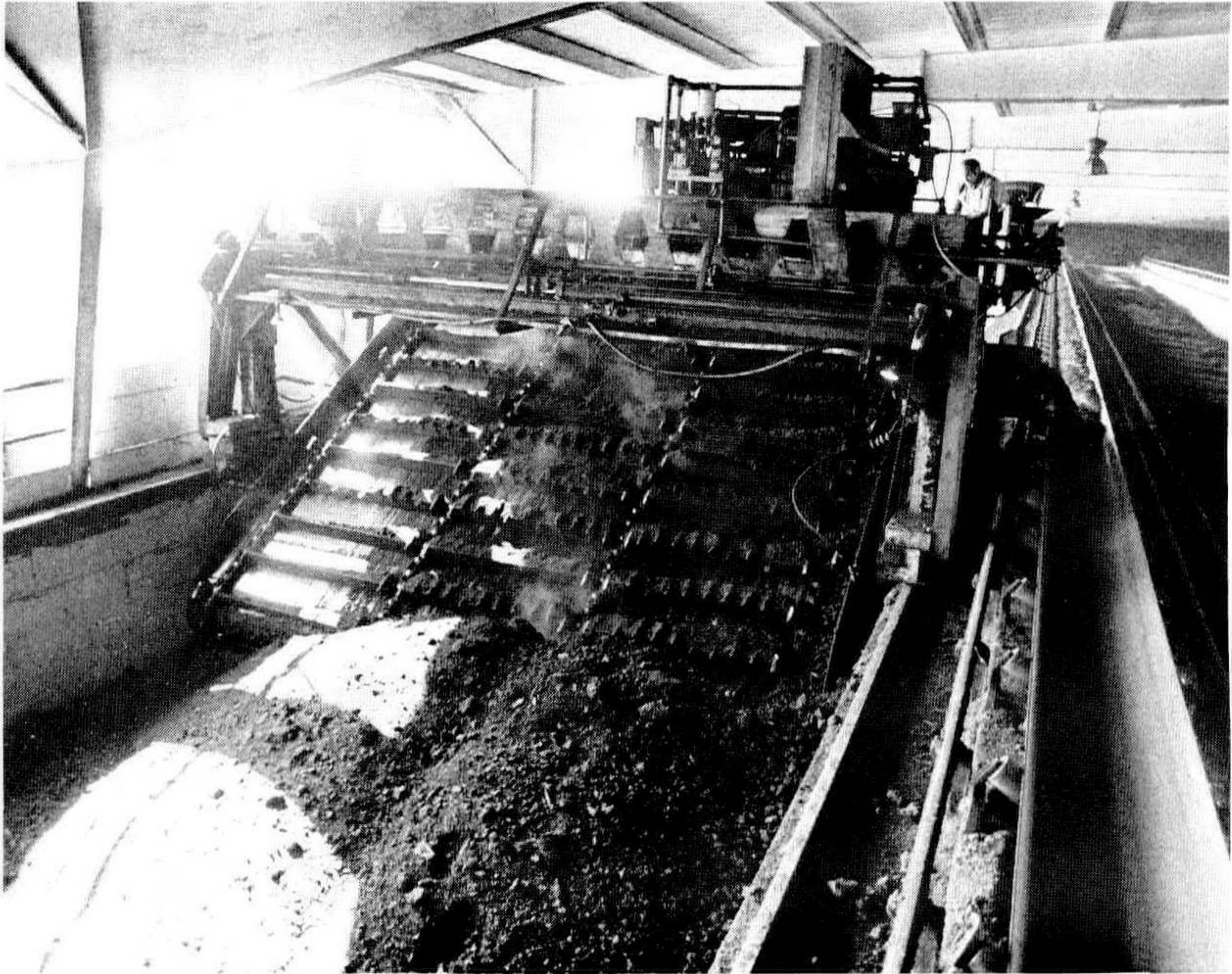
Figure 1. Compost being removed from an aerated bioreactor tank and placed onto conveyor belt. The compost is aerated by fans through perforated floors and turned frequently to expose all organic matter to thermophilic conditions. Tank ( 4 \times 7 \times 150 m) on left filled with cow manure and on right with hardwood bark.
